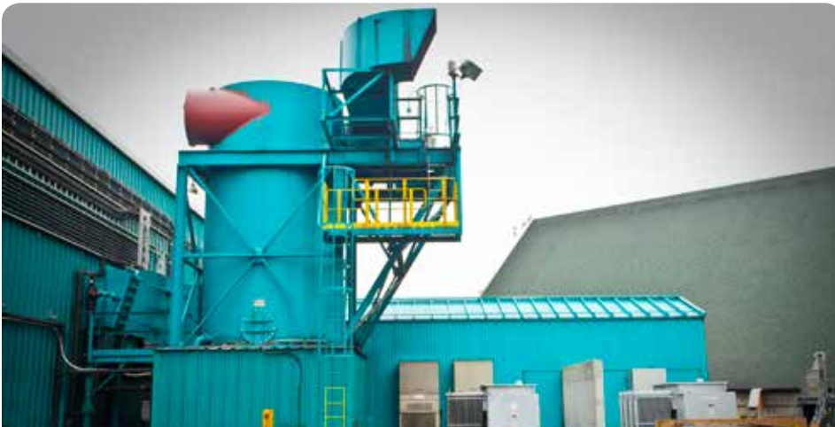
Our scrubber helps keep the steelmaking coal we handle on site.
