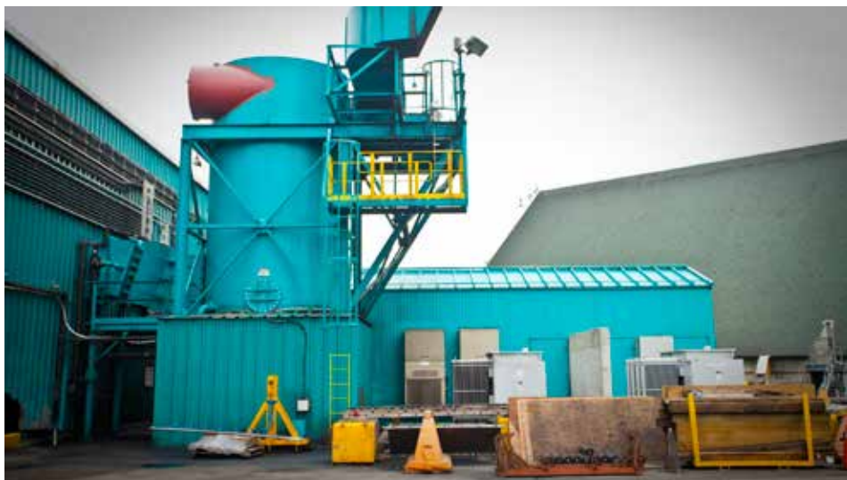
The wet scrubber (above) acts as a huge vacuum for the building and helps ensure dust does not escape and leave the terminal site
